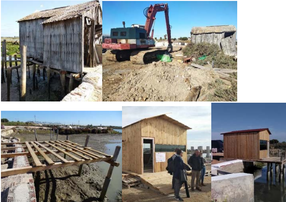
Figure 141. The old mill building before restoration, during reconstruction works and after the intervention (front and back). Salina San Vicente, Cádiz, Spain. ©Salina San Vicente (top left and middle), H.Clavero (top right and below)
