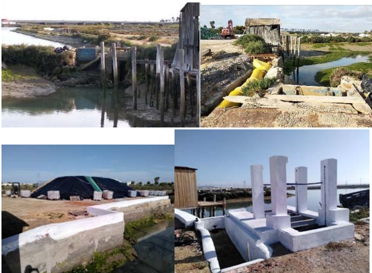
Figure 142. Wall and sluice gate prior to the intervention (above) and after the reconstruction (below). ©Salina San Vicente (above) and H.Clavero (below)
