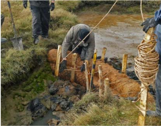
Figure 20. Installing “salt marsh sausages” of coconut coir to try to stabilise degrading coastal habitat. Image courtesy of Essex Wildlife Trust
