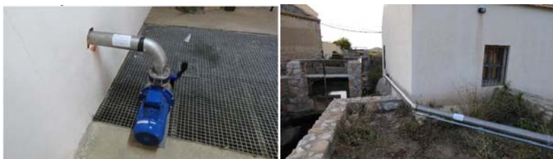
Figure 144. Water pump installed at the Marchamalo salinas, Region of Murcia, Spain. ©ANSE
