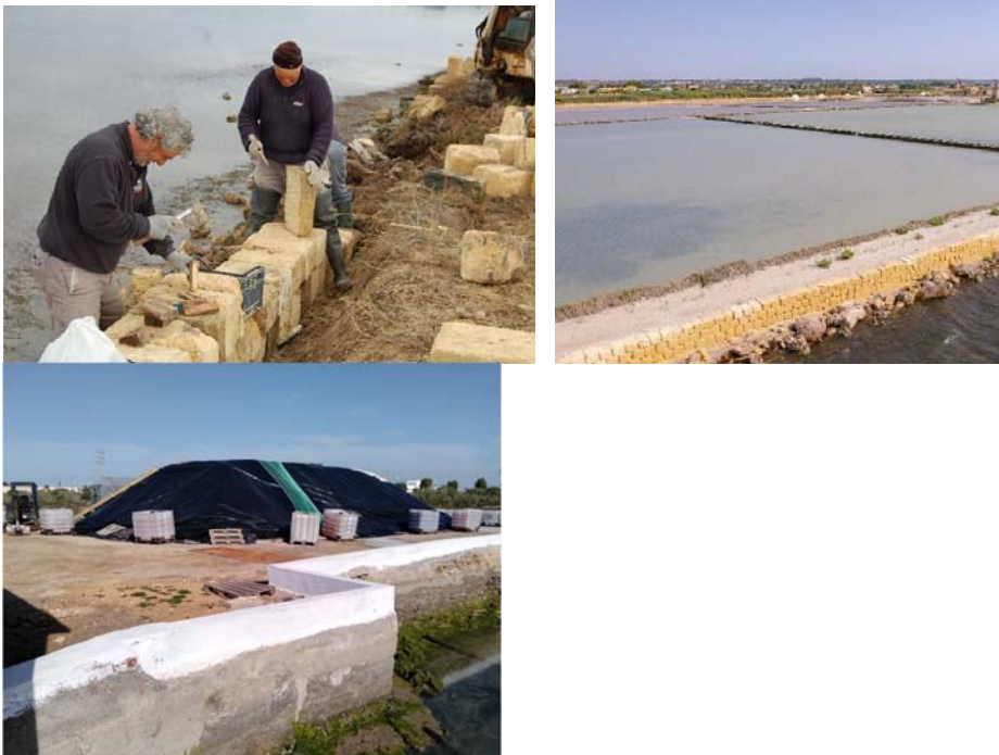
Figure 19. One of the embankments recovered in the Ettore and Infersa salina (Italy) within the MedArtSal project pilot actions (above) and the rebuilt and reinforced wall in the San Vicente salina (Spain; below). ©MedArtSal project
