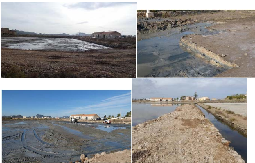
Figure 147. One of the salt ponds (crystalliser) before the intervention (top left), during the works (top right) and once cleaned (below left). The perimeter of the entire crystalliser has been rebuilt (detail of the wall, below right). ©ANSE
