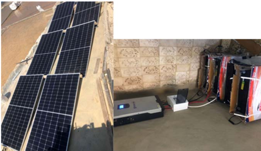
Figure 168. Solar energy production system implemented at the saltworks. ©Imad Malek/Malek Salinas
