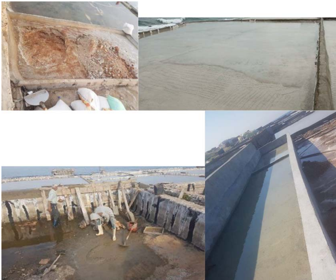
Figure 163. Salina pond rehabilitation (top, and bottom left). After work (bottom right). ©Georges Sleiman/Evaura
