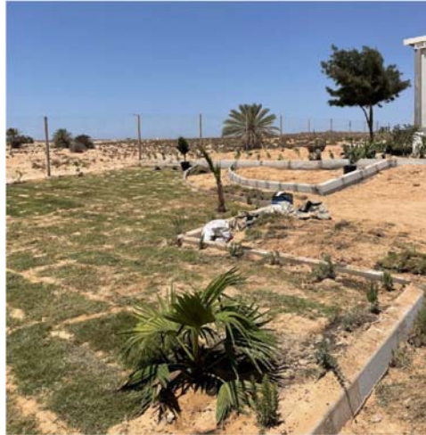
Figure 102. Setting up of the Eden Garden for future events – salina of Sabkhet Lâadhabet (Tunisia) – MedArtSal pilot action. ©MedArtSal project
