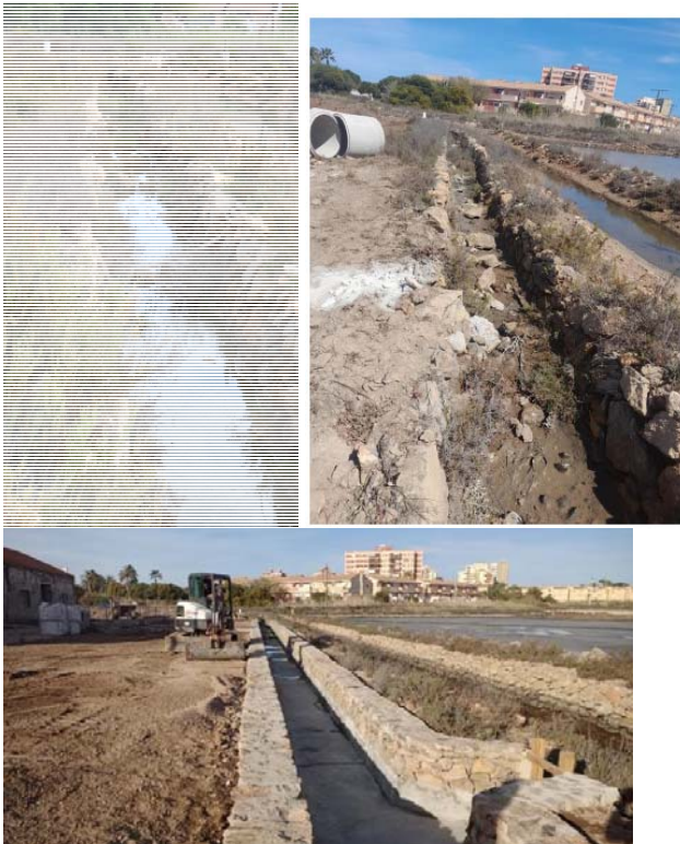
Figure 145. The salt pan's canal before the intervention (top left); during the renovation (top right) and after the renovation work (below). ©ANSE
