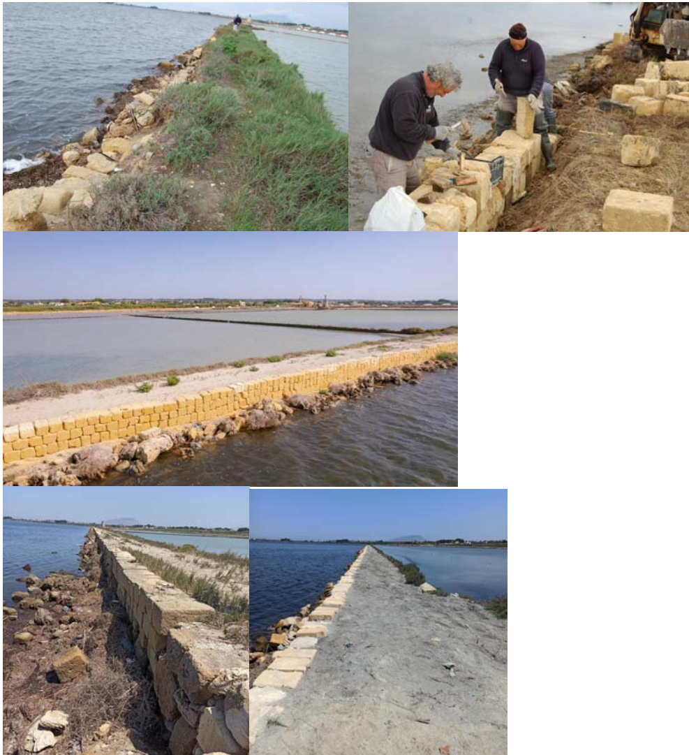
Figure 154. The salt pan's external wall before the intervention (top left); workers at work during the embankment renovation (top right); the embankment after the recovery (middle); details of the embankment (bottom). ©Salina Ettore e Inversa
