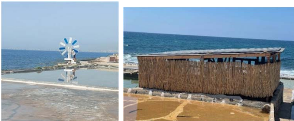
Figure 21. Traditional windmill repaired in Sleiman Sleiman Salinas (left). Solar panels installed in George Sleiman Salinas (right) (Lebanon, MedArtSal pilot actions). ©T.Campisi (left) and MedArtSal project (right)
