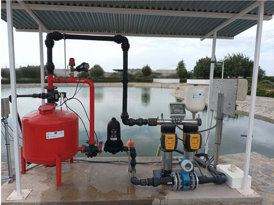
Figure 13. General view of the filtration treatment (pressure sand filter followed by mesh filter) and pressure group.
