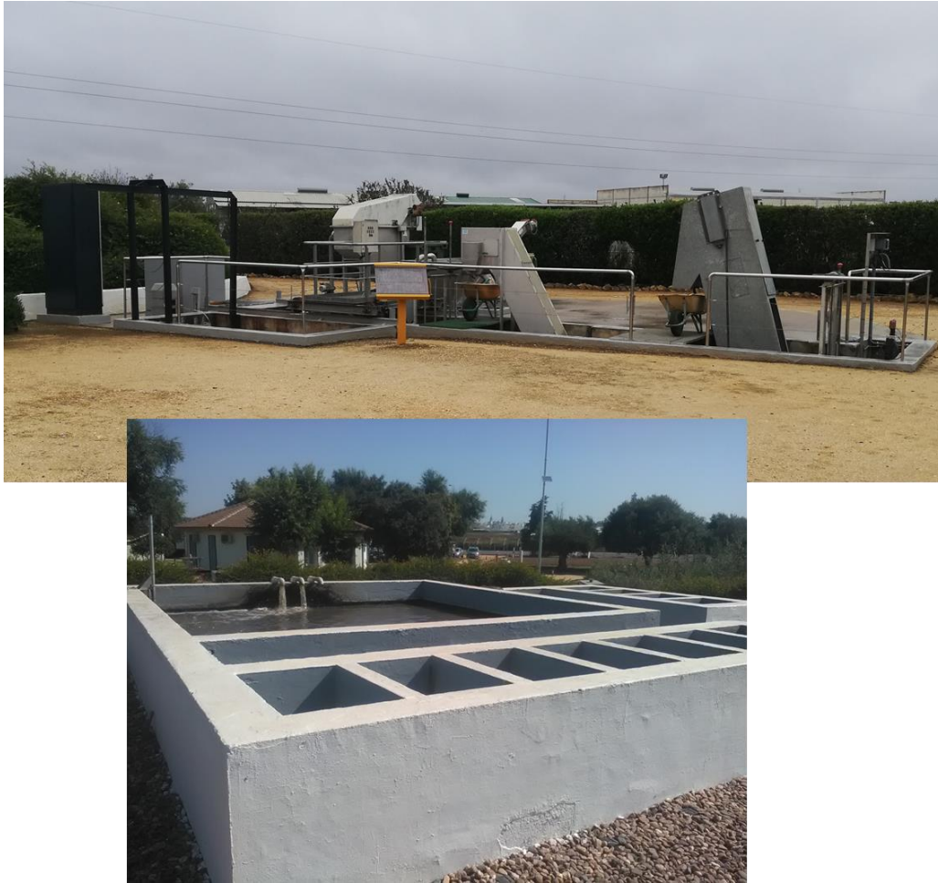
Figure 3. General overview of the pretreatment, homogenization and distribution tank outlets.
