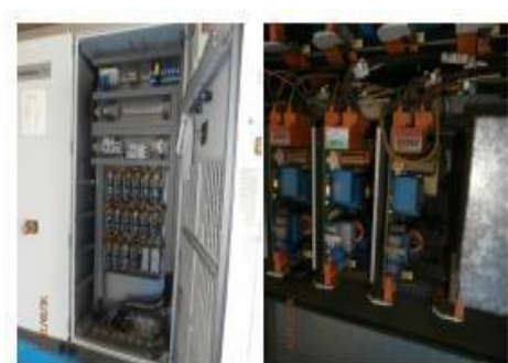
B. Electronic ballasts and the control
