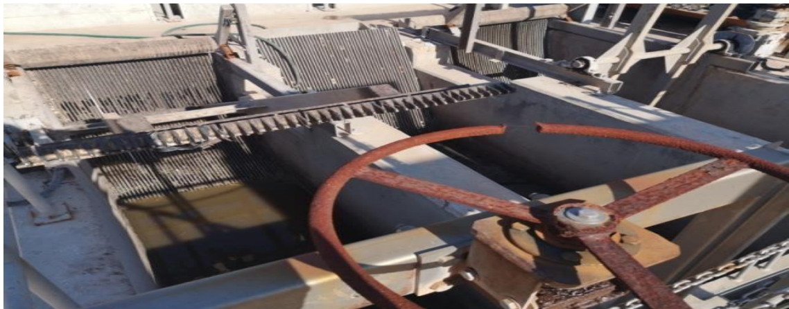
Figure 4. General view of the Preliminary treatment and automatic Screen
