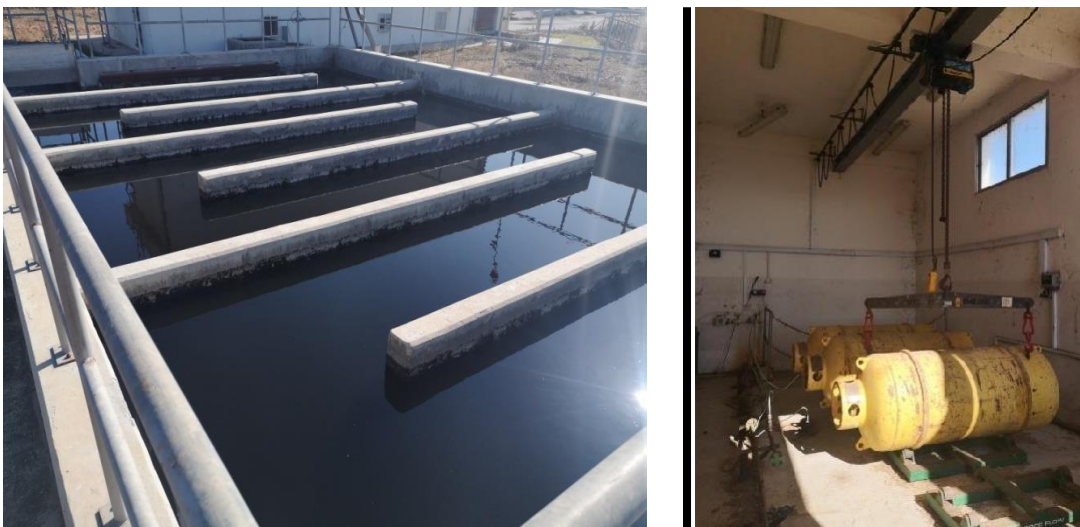
Figure 11. Overview of the Disinfection unit (Chlorination Channel) and chlorine gas containers
