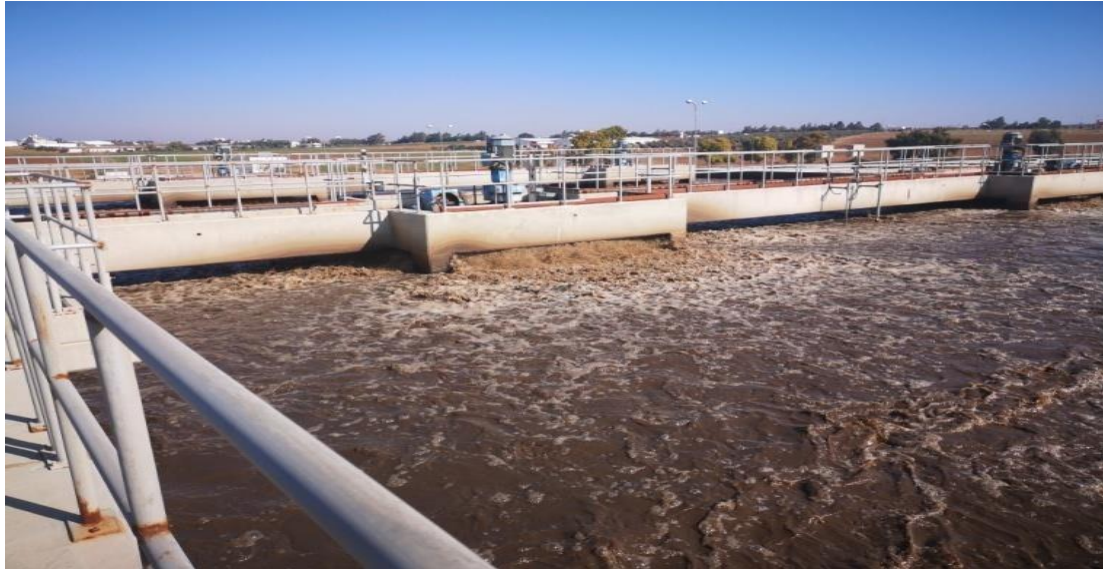
Figure 6. Overview of one of the two Aeration Tanks
