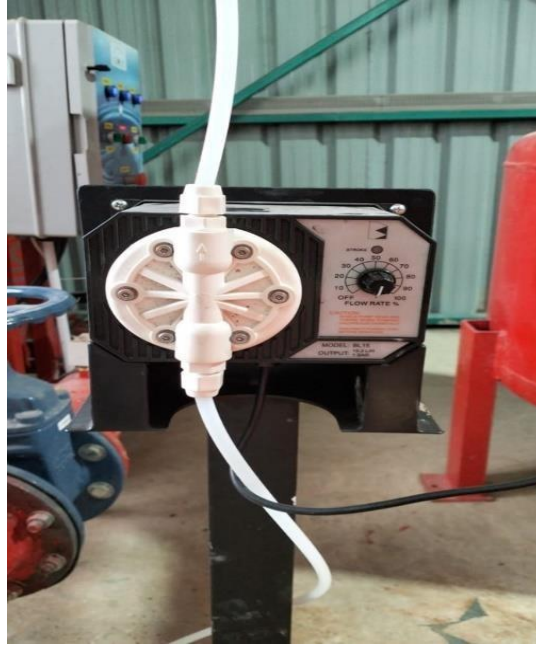
Figure 16. Dosing pump for the addition of hypochlorite.
