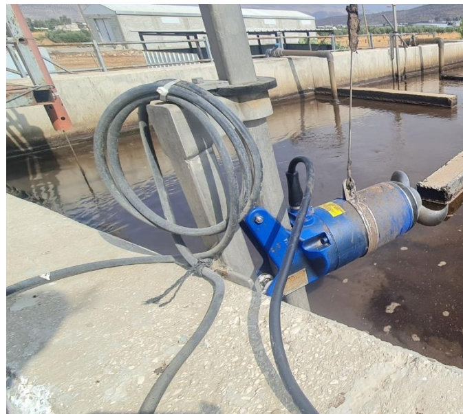
Figure 5. New installed submersible mixer in the aeration tank at Beit Dajan WWTP.
