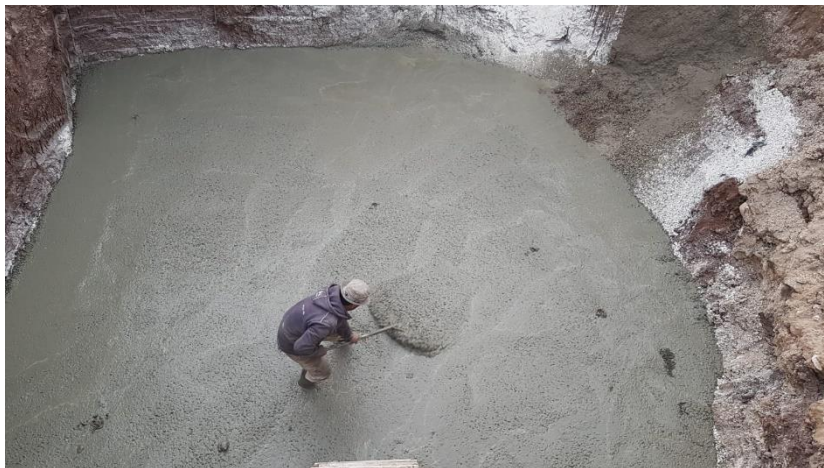
Figure 6. Foundation works for construction of the equalization tank in November 2021 at Beit Dajan WWTP.
