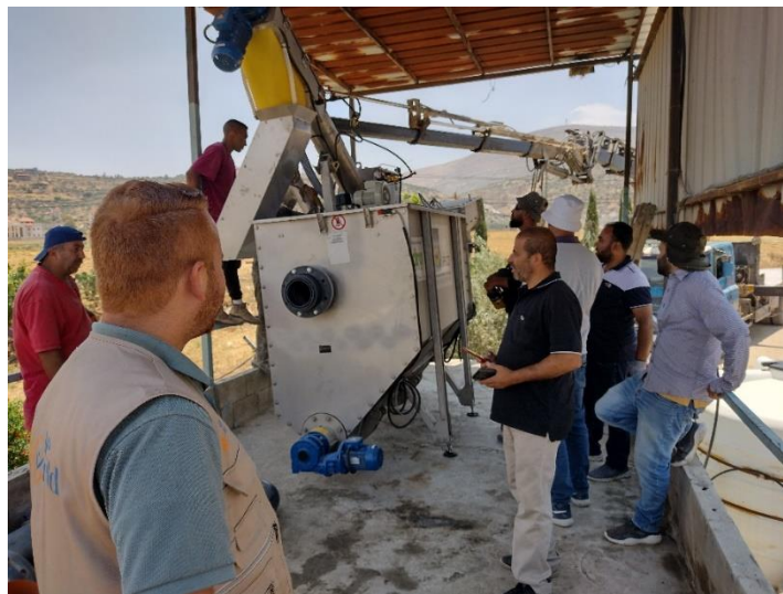
Figure 4. Installation of the pre-treatment unit at the Beit Dajan WWTP on the 7 th of June 2022.
