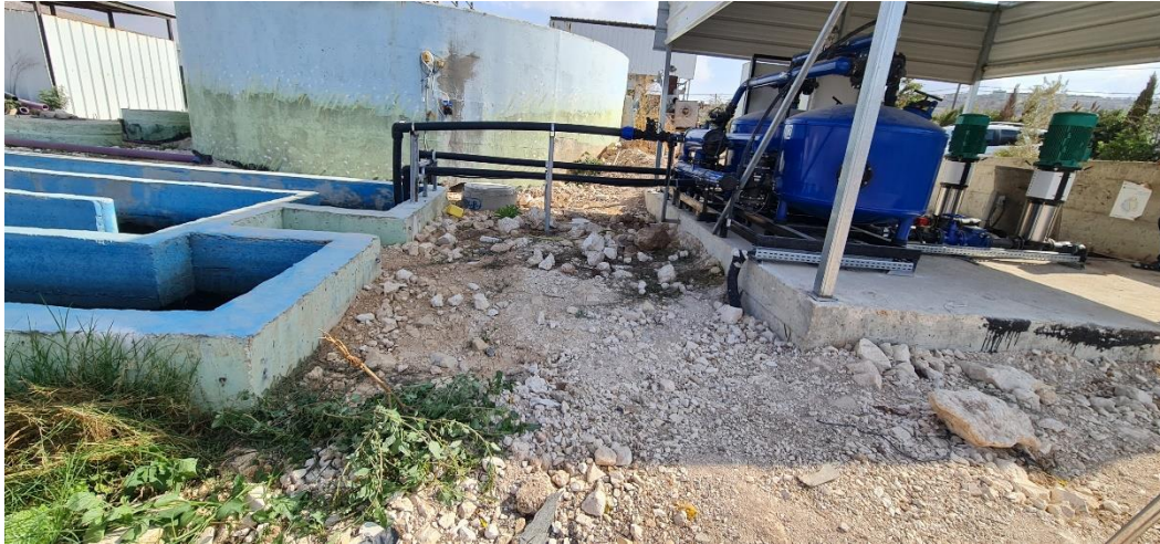
Figure 7. Sand filters installed on top of the equalization tank and connected to the chlorination unit.
