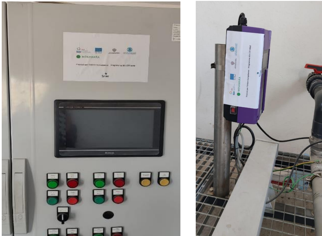
Figure 11. Details of the pumping station
