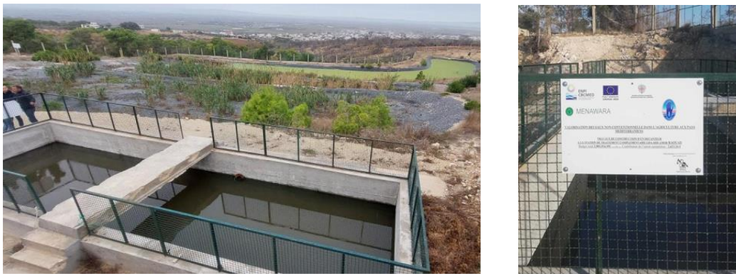
Figure 13. The settling tank and the CWs
